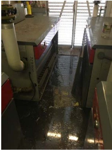
Image showing Stallingborough Failed Boilers in Boiler House
