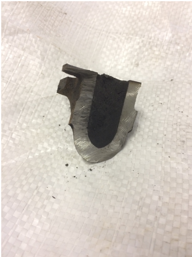
Image showing debris in heater section taken from the Modular Boiler at Stallingborough
